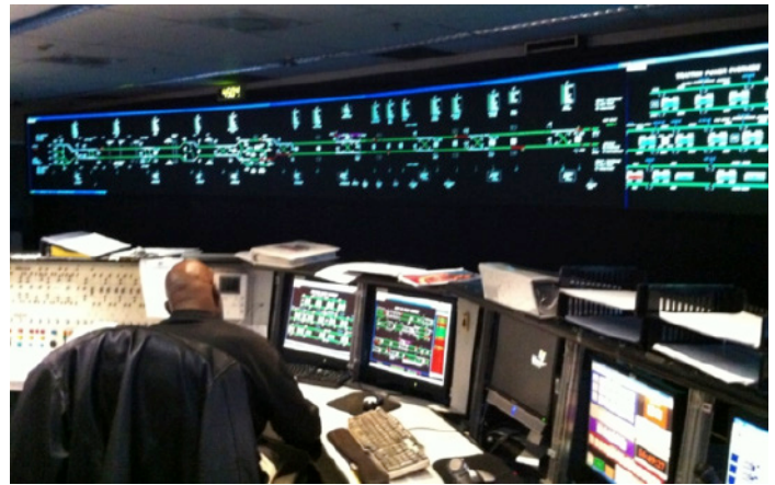
Figure 3. The metro subway control room inside the Maryland Transit Administration (MTA) Control center (4)
